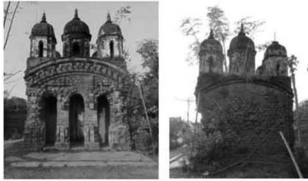
Vandalism noted in late 19th-century temple, Joypur, Bankura. Source -Author
