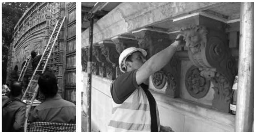
Repair works in the temple in Kendu, Bardhaman. Source- Terracottar Khoje' and Repair work in Central London. Source - Ttie Nolans Group, Dublin
